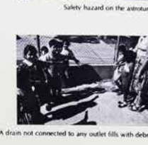
A drain not connected to any outlet fills with debris
